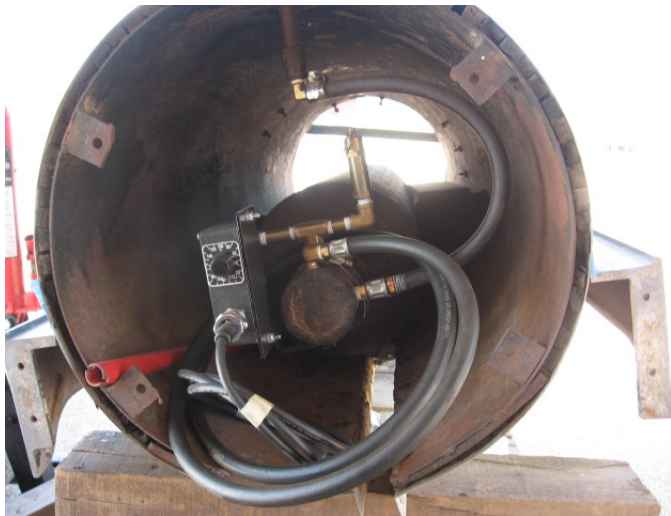
(so that's what's inside a boiler)
